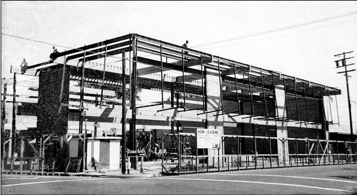
4.16. The Brinley Building under construction, 1963. While not easily readable in this reproduction, the black sign on two white posts at the corner in front of this structure reads “BUSINESS DISTRICT.” An arrow under these words points to the right. This is to say, as late as 1963 the idea that a few blocks on G Street was the business center/downtown was still active at least in the sense that a sign that said so was still tolerated. The building behind that sign, though, told of a rapidly changing reality. (John Weber Brinley.)
