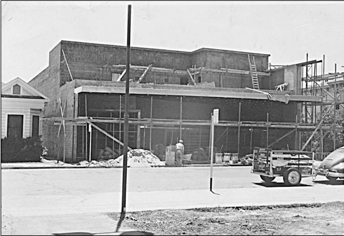
4.5. The Varsity Theater Under Construction, 1949. In the late 1940s, the Luft's sold the original Varsity Theater at Second and F to Westside Valley Theaters and also sold that company land west of their house on which Westside then built a new, "state-of-the-art" movie house with the same name. On the left we see the Luft home still in place and the new theater under construction. At this same time, the original Varsity was demolished. (Phil Brady.)
