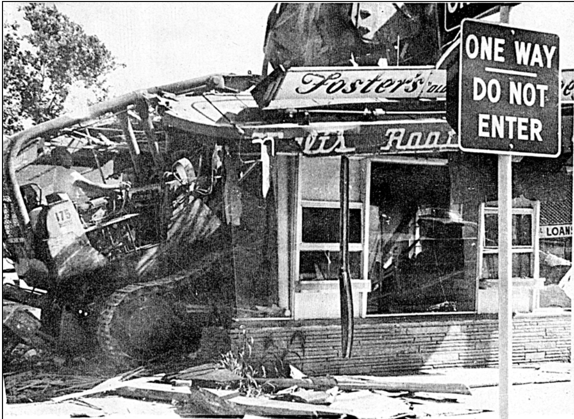
FEW TEARS SHED — Foster's Freeze at the corner of Second and F Streets, for 17 years a favorite place for a quick sandwich and the number one spot in Davis for girl watching was demolished early today. Clay Quessenberry, owner of the property will erect a modern two story building on the site. Shown operating the bulldozer is Roy Nielsen of Nielsen's Demolition Contractors of Sacramento. — Enterprise Photo
